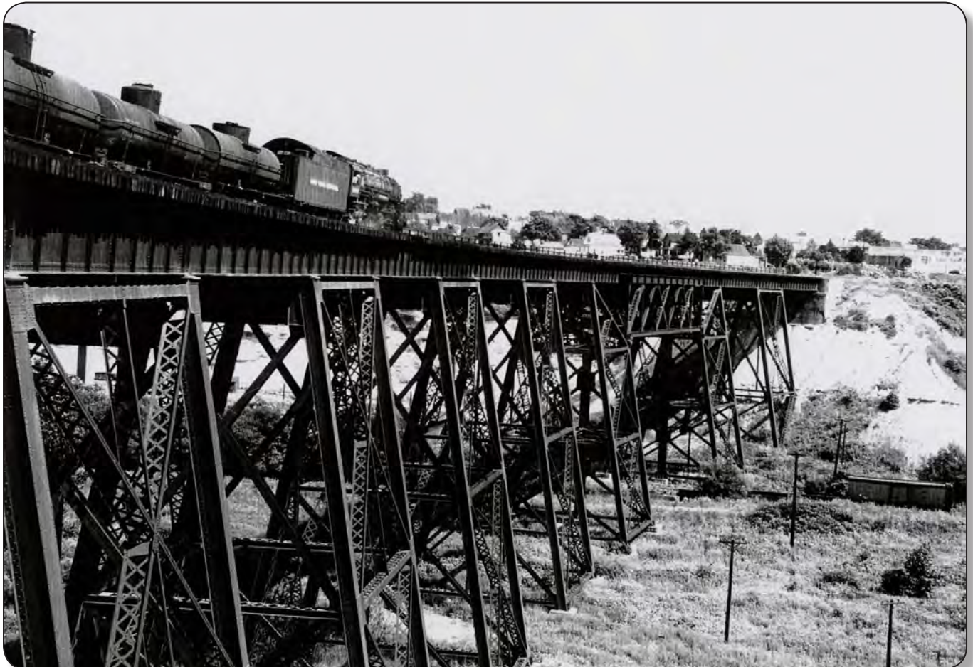
Lake Erie and Pittsburgh Railroad trestle over Mill Creek, Cuyahoga Heights; utilized by New York Central in 1948 (Albert C. Doane).
