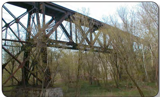
Lorain & West Virginia Railway trestle over the Black River in Sheffield; railroad traffic over the trestle was abandoned in late 1960s. View of the trestle over from Lorain County Metro Parks' Bridgeway Trail, Sheffield.
