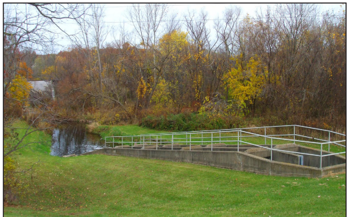
Outfall structure on French Creek at the end of the treatment process, where up to 5 million gallons of water are discharged to the creek each day.
