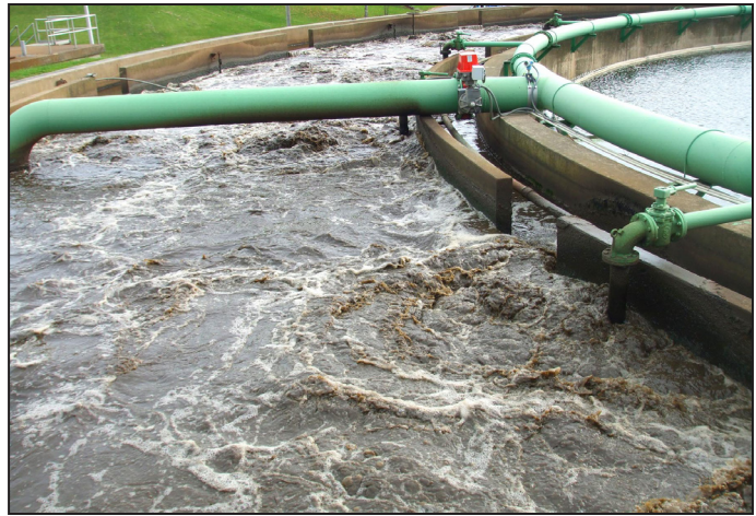
Primary Clarifier Tank where aeration separates and microbes digest sludge in the outer ring. Sludge is deposited in the quiescent waters of the center ring.
