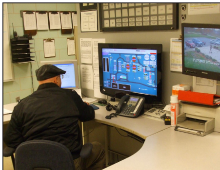
Control Room in the Administration Building where the processes in the plant are monitored and controlled.
