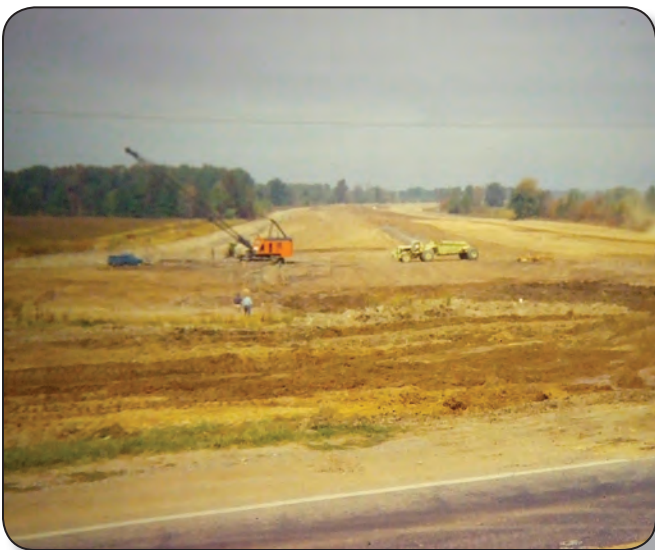
Construction of I-90 interchange at SR 254 in 1966 (view to the north), which required the widening of Detroit Road.
