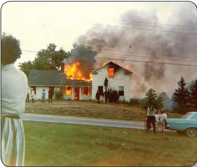
Edward Brown house being burned in 1966 to accommodate widening of Detroit Road.
