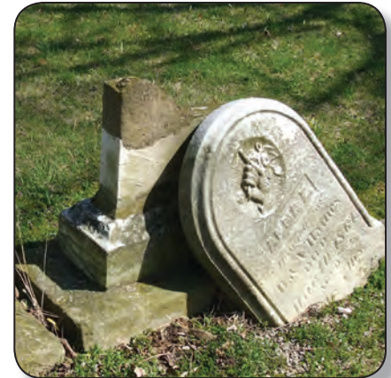
Example of damaged grave marker—Haines Family in Block B of Garfield Cemetery.
