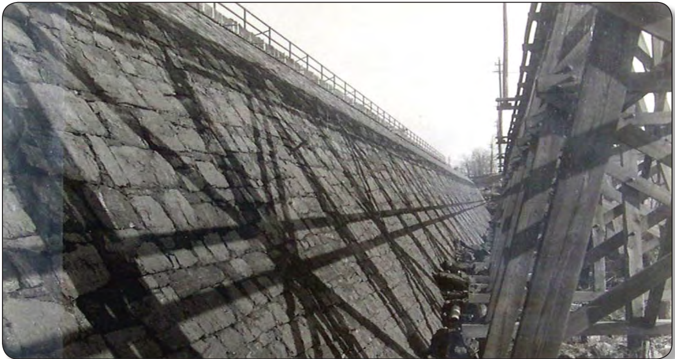
Causeway construction for the East 31 st Street bridge in 1913 showing timber supports for 1905 Avon Beach and Southern electric railway trestle (Black River Historical Society).
