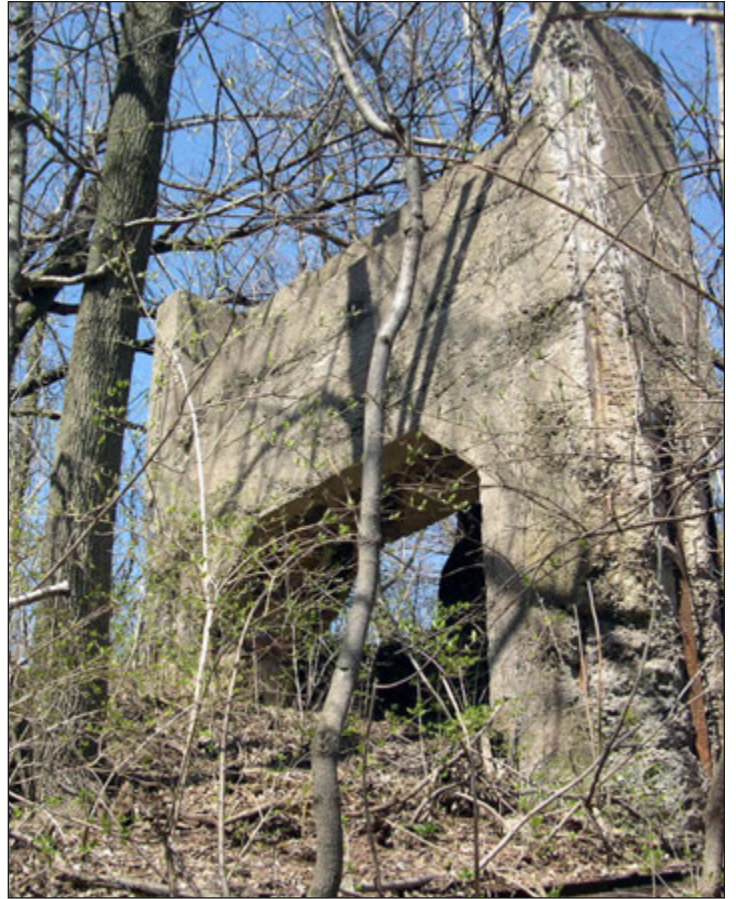
Abandoned concrete pillar of the 1905 Avon Beach & Southern electric railway trestle over the Black River at East 31 st Street as it appeared in April 2008.
