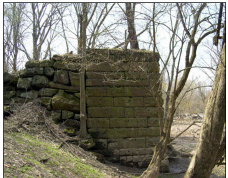
Abandoned south approach to Days Dam bridge as it appeared in April 2008.
