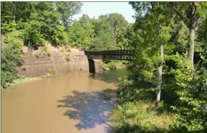
1,000-foot-long Bridgeway Trail double bridge over the Black River in Sheffield. Photograph taken from the upstream span of the bridge.
