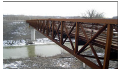
Crossing French Creek near its confluence with the Black River, this new Metro Parks' bridge is part of the two-mile Steel Mill Trail opened May, 10, 2008.
