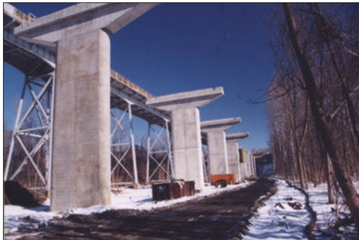
Concrete pillars for construction of new Garfield Bridge with original Garfield Bridge in the background at left in 2000.
