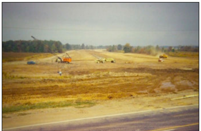
Construction of I-90 interchange at SR 254 in 1966 (view to the north), which required the widening of Detroit Road.
