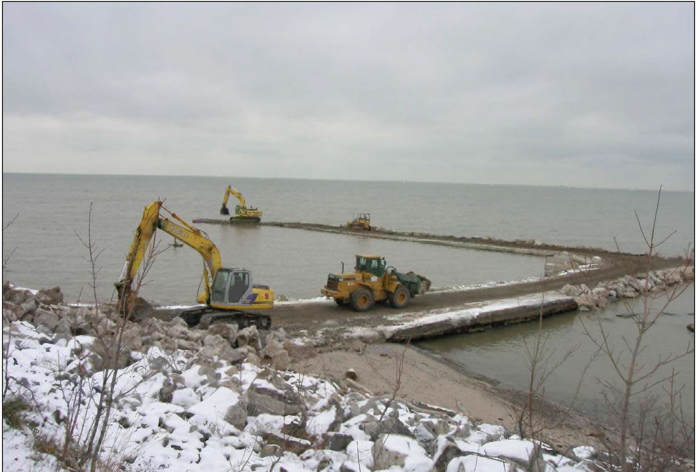
Sheffield Lake Community Park marina, at the head of Lake Breeze Road, under construction in December 2007. The marina includes a boat launching ramp and associated breakwaters to protect the ramp from wave action.
